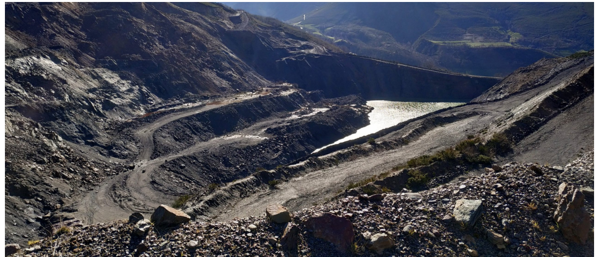
Mine of Tormaleo in Asturias, where mine restoration is occurring. Native vegetation will be recovered, along with a lake, and trails are being built together, creating a region that is ecologically healthy and will support tourism.
