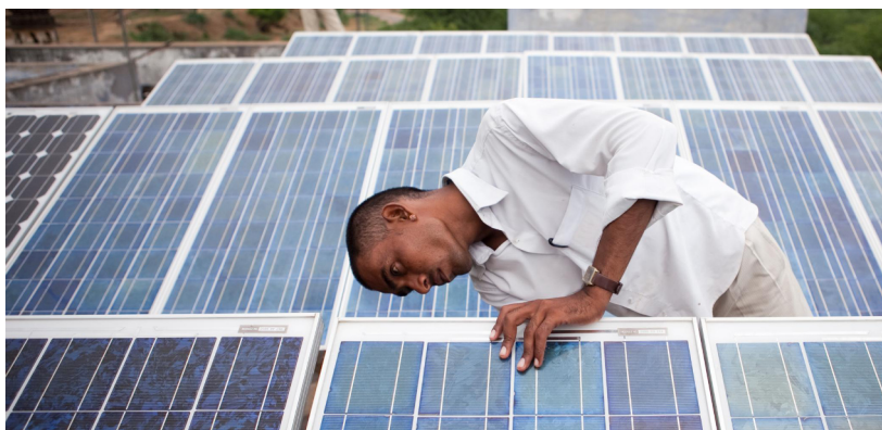
Parama Ram, 23, maintains the solar panels that power the water desalination plant in Kotri Village, Rajasthan. The plant produces over 3000 litres of drinking water per day. Before the plant was installed, the villagers would often have to drink the salty groundwater. Photo: © Prashanth Vishwanathan/Greenpeace
